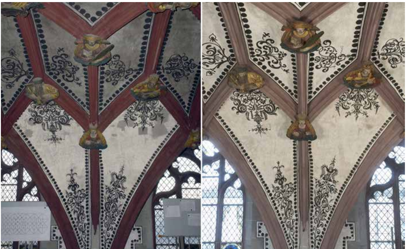
Fig.8: Intermediate state of an exemplary axis in the choir vault: partially cleaned with visible grey retouching from 1910 (left) / final state after cleaning and painting over the vault ribs (right). 2015 / 2017, Berner Münster-Stiftung.
